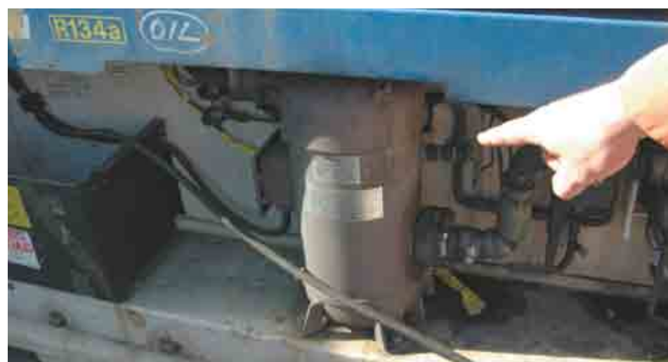
Potentially dangerous: Container companies saved money by using cut-rate contractors in Vietnam to service refrigerator compressors like this one. The decision led to the deaths of three dockworkers and triggered an expensive global safety problem when compressors began exploding.
